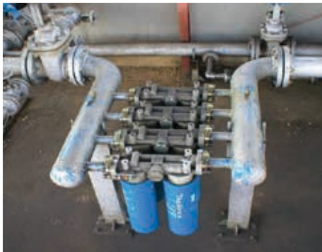
Single-pass Bulk Fuel Filtration System
